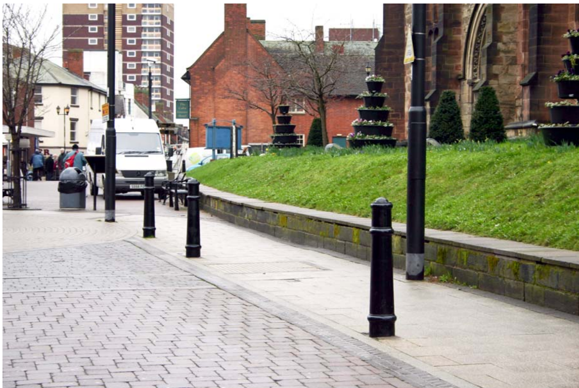
Poor-quality concrete slab coping to dwarf wall around church precinct and inappropriate planters on bank
