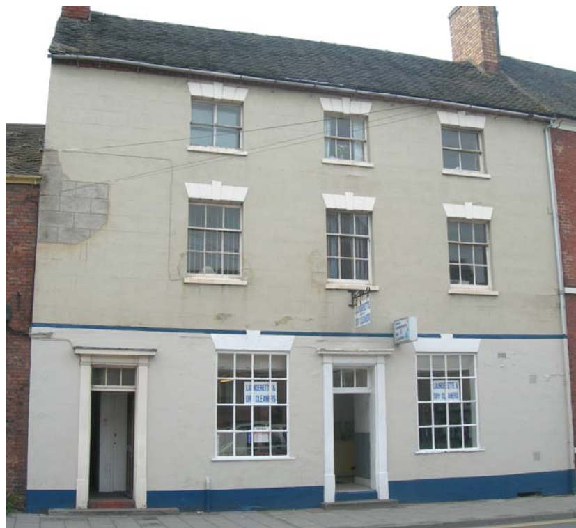
The listed Nos. 20-21, in need of some maintenance to its façade
