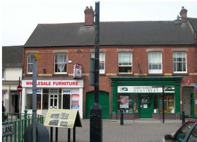
Nos. 23-25A Lower Gungate, recommended for local listing. The detrimental impact of street furniture is apparent
