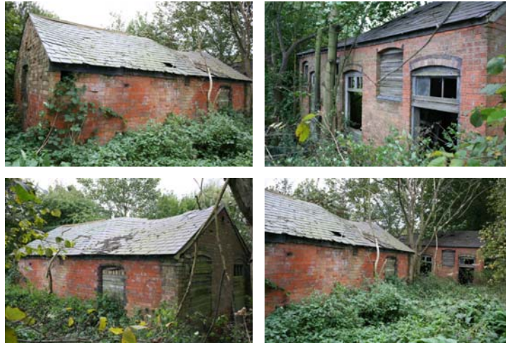
The outbuildings in need of attention
