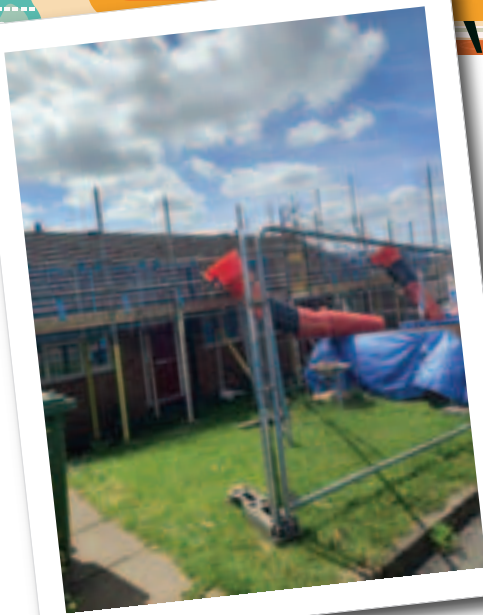
Roofs at Edward Court (Before)
