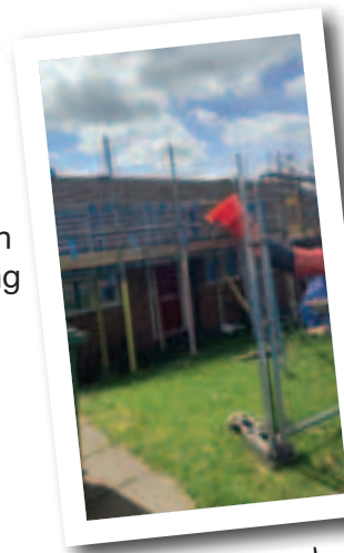
Roofs at Edward Court (Before)
